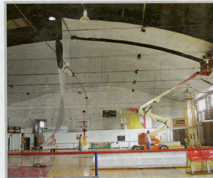
Metal buildings have very large wall expanses, open areas and are not typically compartmentalized like other types of commercial buildings, which heighten the need for fireproofing. (Photo courtesy of RIMA International)
