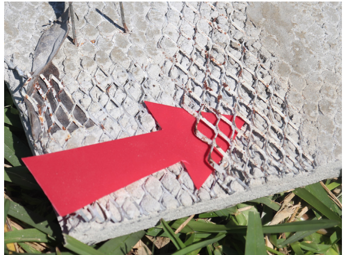
This image shows areas where the lath has been fully embedded on all sides by the stucco—as well as areas (red arrow), where the lath is fully free-floating, with no embedment. The areas where embedment is insufficient are prone to issues from moisture penetration and corrosion.
