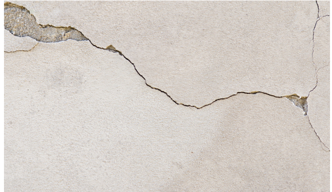
These cracks are likely stucco curing-related, but also could be related to lack of lath embedment.
