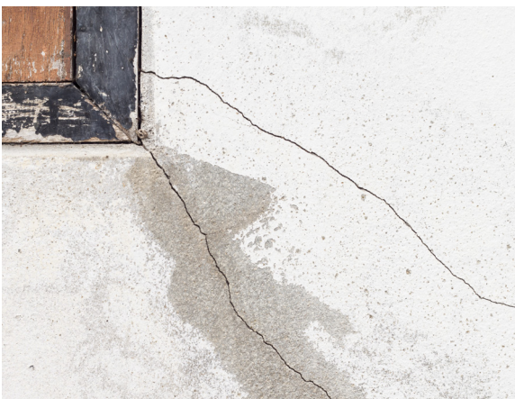
Stress-cracking often seen in corners can be caused by poor embedment, or omission of control joints placed for stucco membrane movement.
