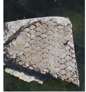
Diamond mesh lath, if not properly embedded in the scratch-coat, may rust and deteriorate.
