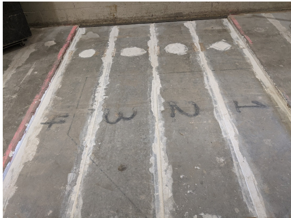
Figure 3 – Concrete slabs prior to installation of carpet flooring, viewed from source room
