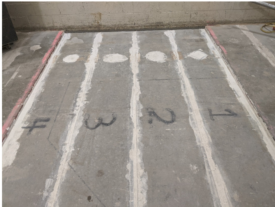
Figure 3 – Concrete slabs prior to installation of LVT flooring, viewed from source room
